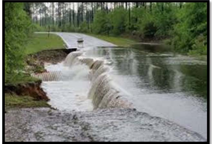
Roadway crumbles along CR3280 at Magnolia Lodge Road in Freeport. Photo courtesy of Walton County Sheriff's Office
