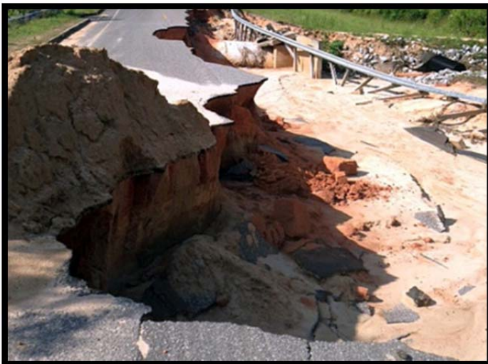
Road washed out due to flooding In Okaloosa County. Source: Crestview Bulletin, Matthew Brown
