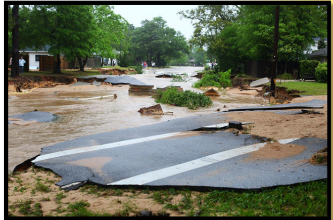
The road bed of Piedmont Street crumbles after it washed out due to heavy rains. Source: Getty Images, Marianna Massey
